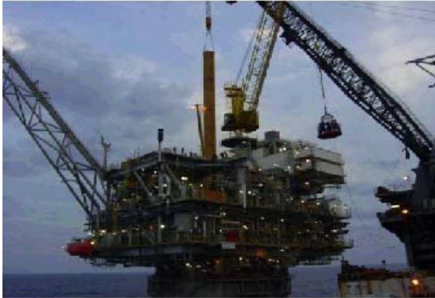
Figure 9 – Spar Aircan Installation
