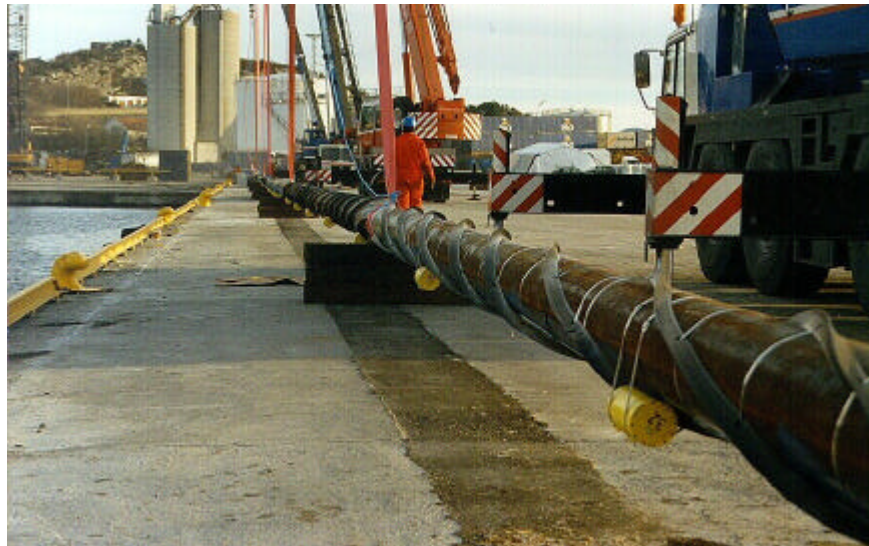
Figure 6 – Strapped on Passive Data Loggers
